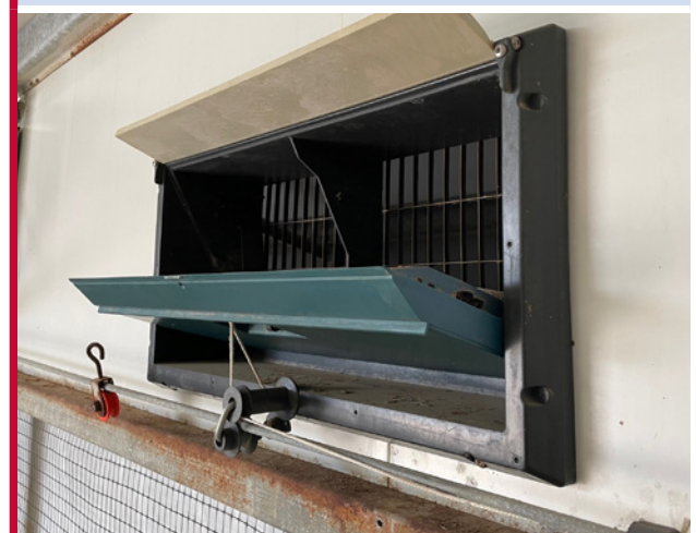
Figure 100 Example of a good-quality air inlet.
