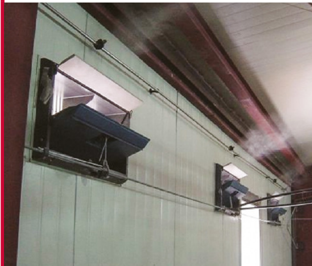
Figure 112 Example fogging system for a cross-ventilated house.
