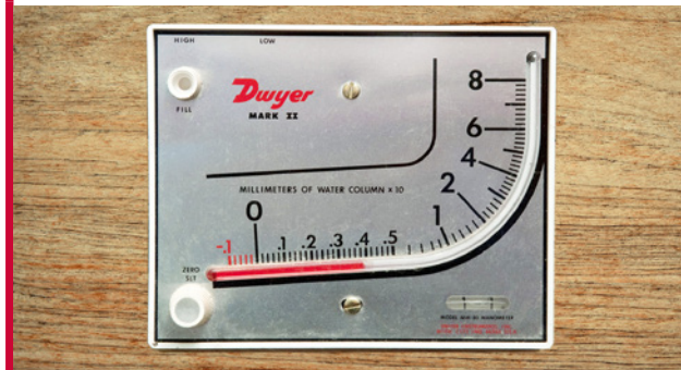
Figure 99 A manometer used to monitor air pressure within the house (the reading given is equivalent to 0.15 inches of water column).
