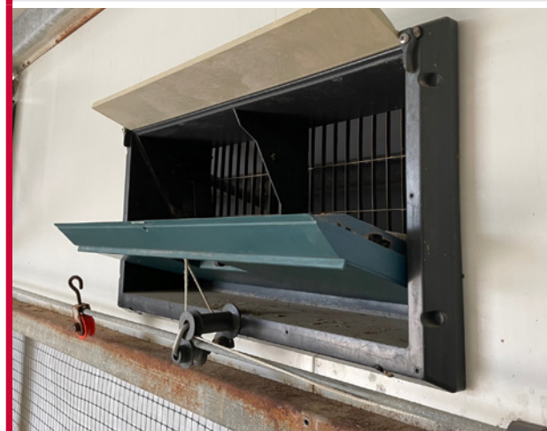
Figure 100 Example of a good-quality air inlet.
